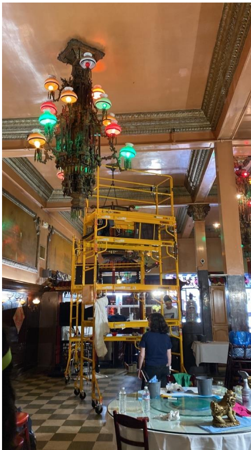
Figures 27-29: start of situ project featuring chandeliers and murals with scaffolding erected.
